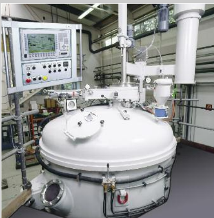
Operator platform with state-of-the-art process visualization
