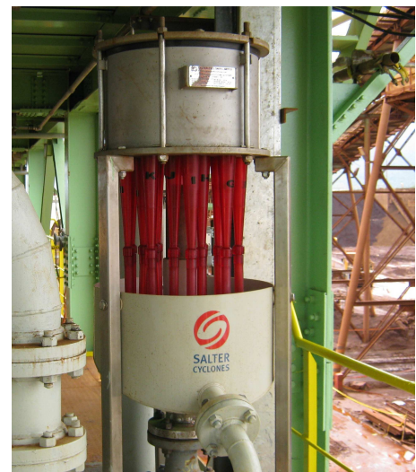
SC2018 - 18 way 2 inch Canister Assembly operating as a pilot unit on site in Far East
